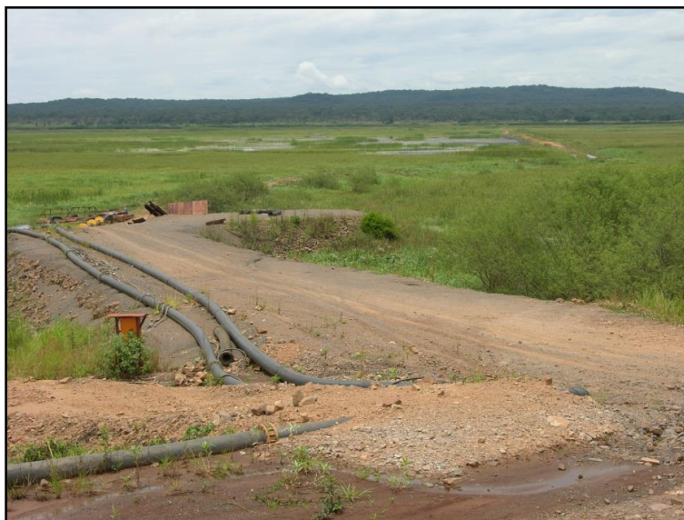
Picture 17: Water pumping station for MUMI plant on the banks of the River Kando (Photo: C.Peyer/BFA)
