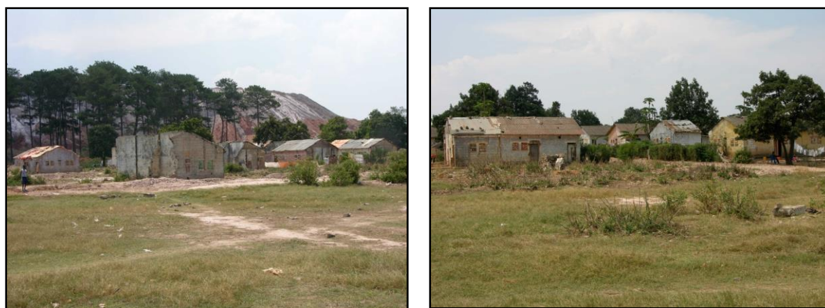
Picture 40: Musonoi: in some parts of the township, mainly the parts which were supposed to be relocated, houses are in a very poor state
